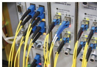
Switches and routers for carrier, access, enterprise networks.
